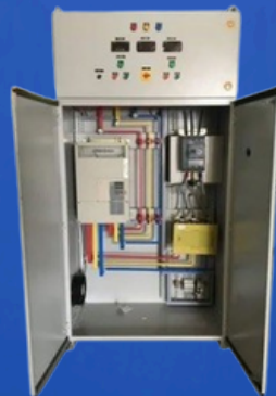
VSD Control Panel
